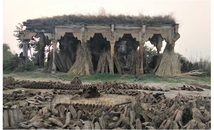
Figure 27 : Sarai in Shahabad, Manikpur Source: Primary survey by AH Division, INTACH Team
