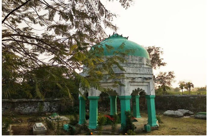
Figure 23 : Hazrat Raje Noor Shah Maqbara, Manikpur Source: Primary survey by AH Division, INTACH Team
