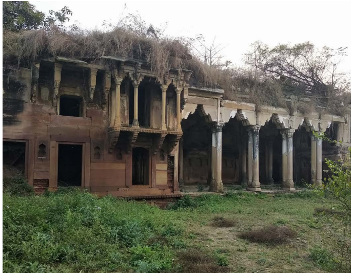
Figure 7 : Raja Taashuq Hussain Mahal, Manikpur. Source: Primary survey by AH Division, INTACH Team
